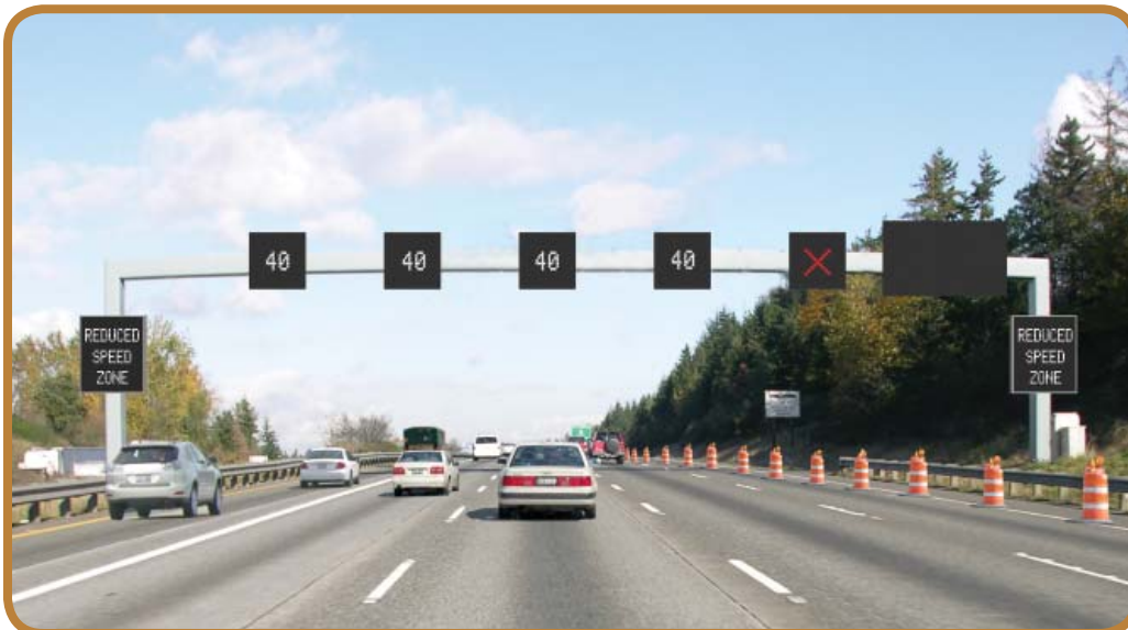
Future variable speed limit and driver information signs will improve traffic flow and safety on northbound I-5 between Boeing Access Road and I-90. Similar signs will also be used in the 520 corridor.
